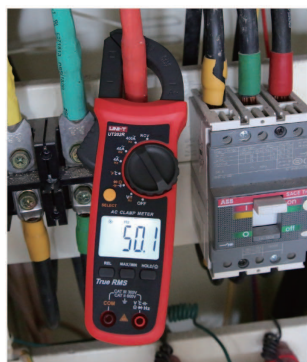
High voltage (600V) frequency measurement
